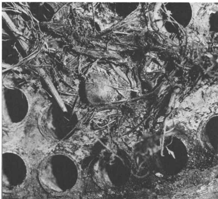
Figure 6. Cooling system heat exchanger partly clogged by aquatic weeds and shellfish
